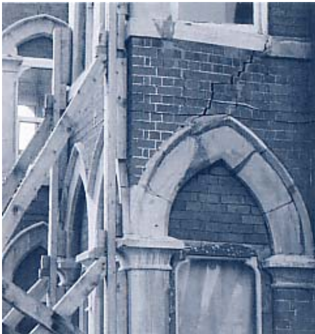
Fig. 9: Structural failure of pointed arch and wall above, due to differential settlement between its two sides. This can often be the result of inappropriate strengthening of part of the foundations.
